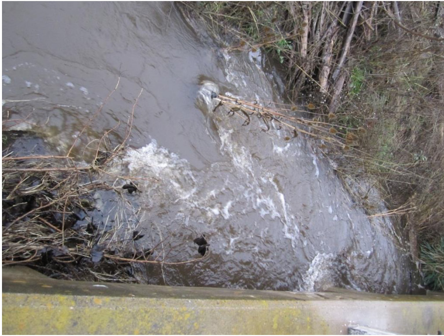
West Sides water entering culverts under Main St.
